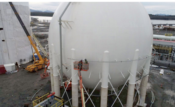
Pembina's new Prince Rupert Terminal includes three above-ground storage spheres where propane will be offloaded from rail cars and stored until it is loaded on ships destined for international markets.
