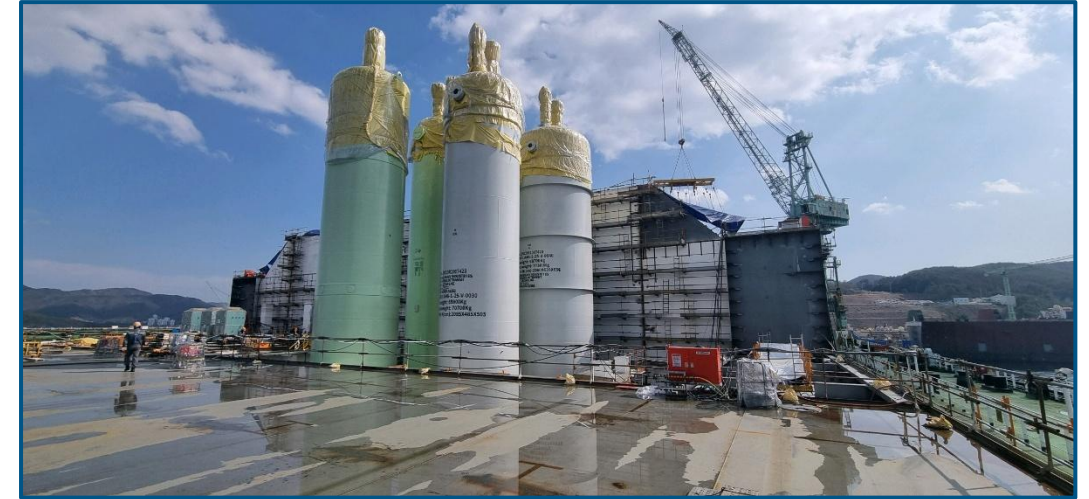
Vessel Top Side and Supporting Infrastructure
